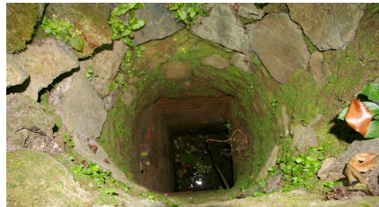
Fig. 14. Access shaft aligned with the underpass at Grotte Renara. Photo: R. Taylor.
