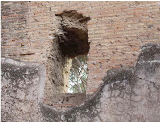
Fig. 15. The opening for the specus in the northern wall of the reservoir.
