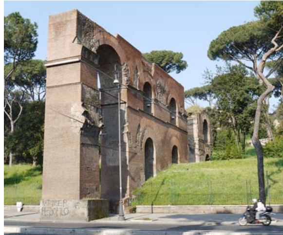
Fig. 19. A view of the pylon near the Via Triumphalis that shows the beginning of two arches on top of each other.
