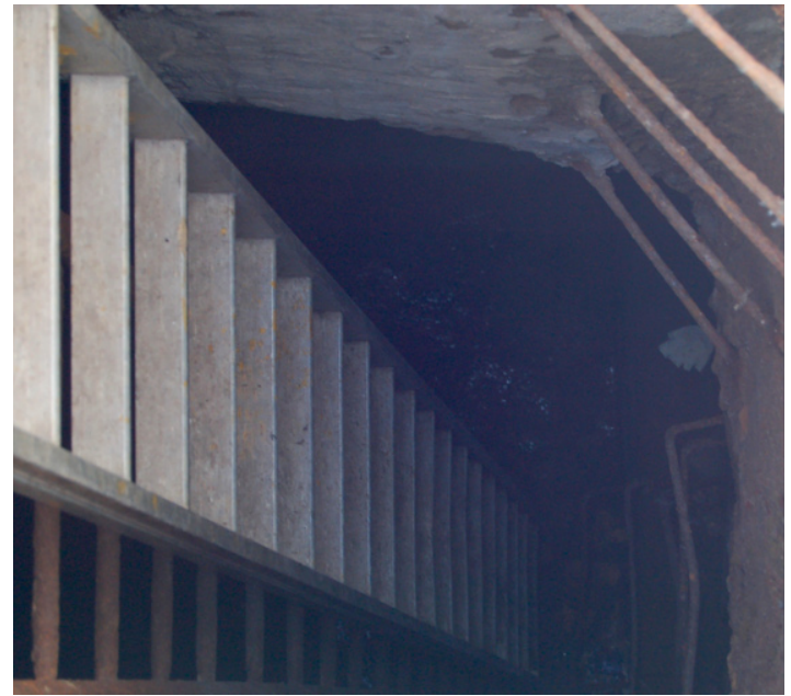
FIG. 16. Cloaca Maxima. View from Forum Transitorium entrance to floor of Canal. Photograph by John N. N. Hopkins
