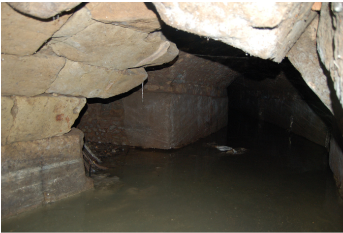
FIG. 6. Cloaca Maxima. Juncture between early-republican, late-republican and archaic tracks, with repairs. Photograph by John N. N. Hopkins
