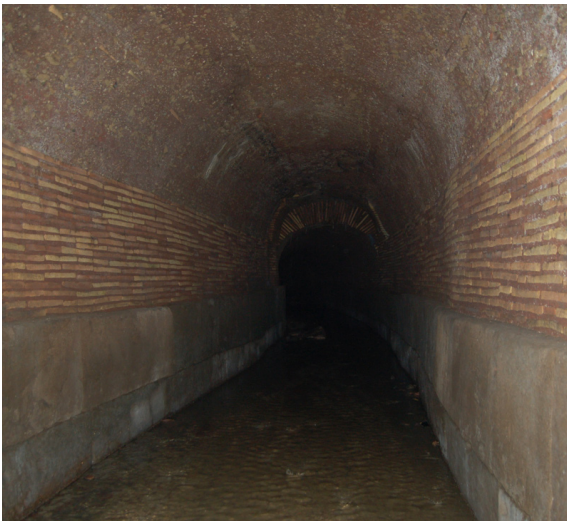
FIG. 8. Cloaca Maxima. Track under Forum Transitorium. Photograph by John N. N. Hopkins
